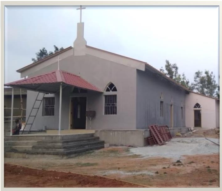
Trinity Edavaka Mission thanks all who supported the construction of a Mar Thoma Shivanapura Mission Chapel at Kalappanahalli village in Kanataka State
